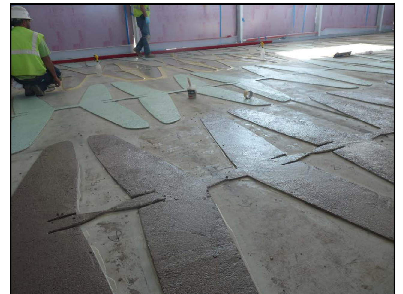
Green and grey terrazzo mixtures have been poured and troweled in place.
