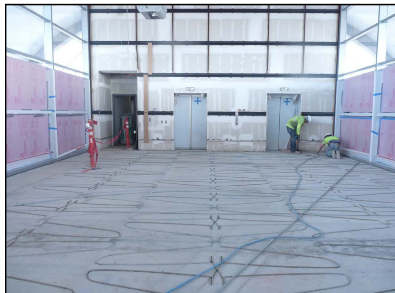
Advance Terrazzo specialists attaching the metal components to the floor. The metal outlines define the various fields of color.
