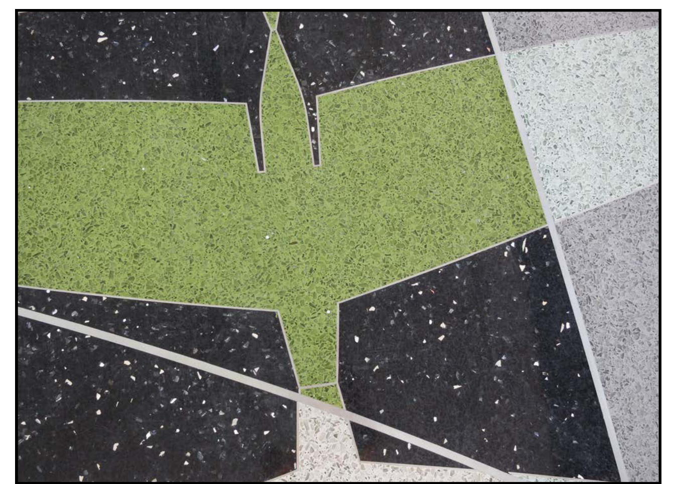
The finished terrazzo floor (detail) after grinding and polishing. The floor's design incorporates ten different colors.
