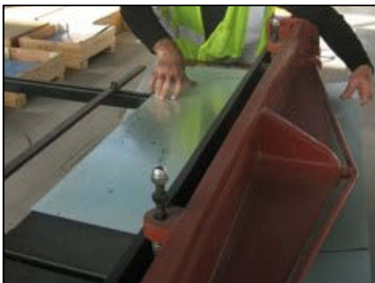
Shearing the aluminum sheet into the reflector panels. Each of the 6,610 panels are uniquely shaped.
